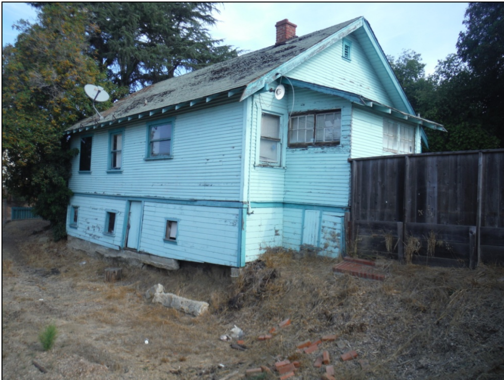
Photo 16. View northeast of 3247 D Street. Undermined foundation on west side evident.
