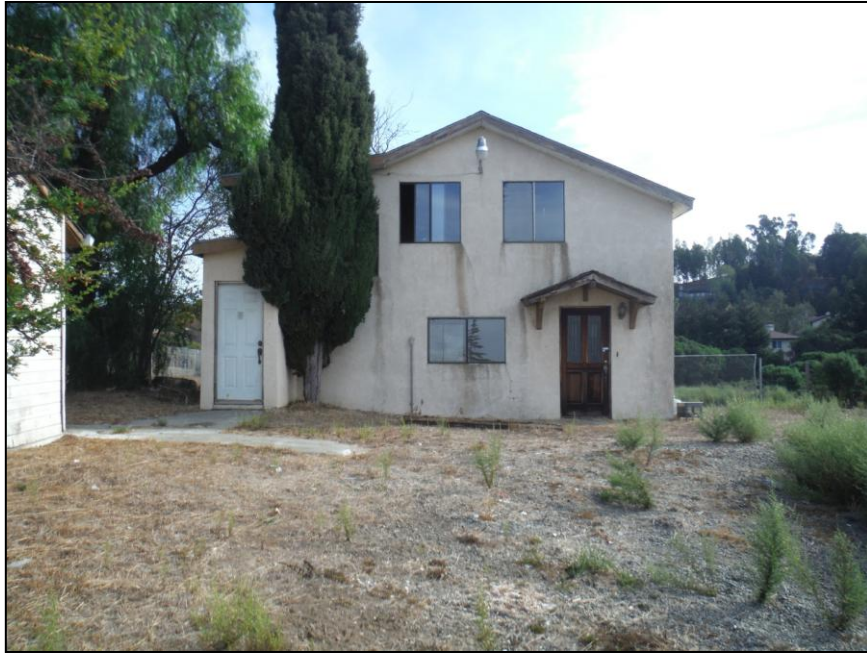
Photo 1. View east of facade of renovated garage (now a residence) at 3291 D Street.
