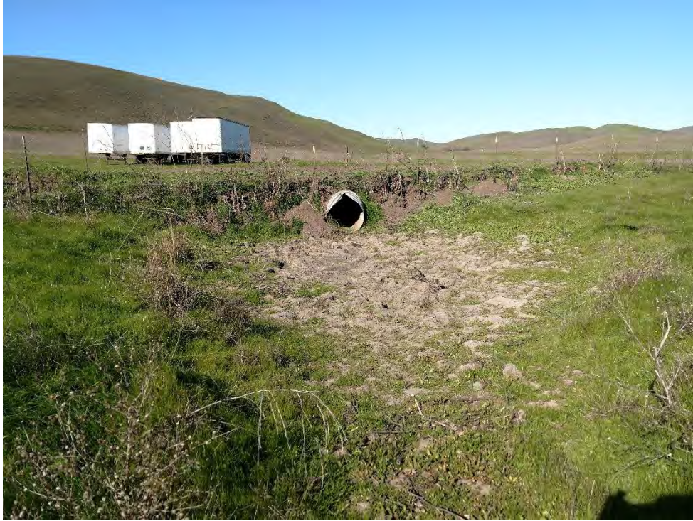
Photo 9. View of the small pool (same feature as Photo 6) below a culvert outfall along Cayetano Creek looking west from west of the southern boundary of the central parcel. Photo date 2/6/2020.
