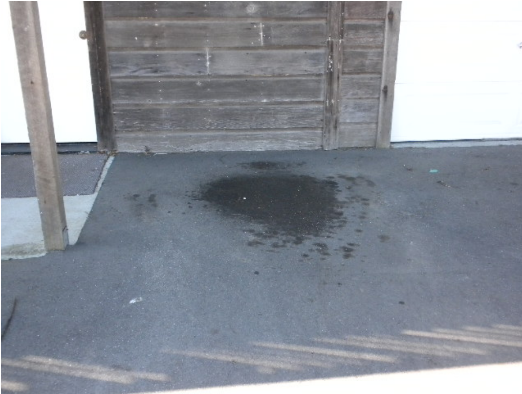
Photo 9: Oil Stain in Front of Garage
